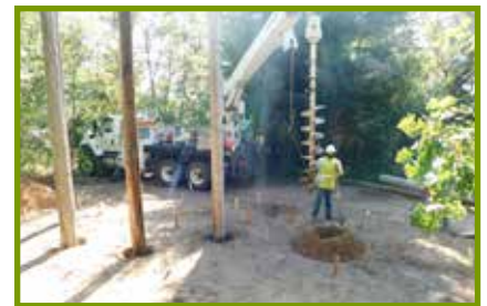
Eau Claire Energy Co-op workers brought a large auger to bore the large holes for the utility poles. Photo by Staff
